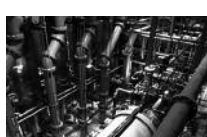
Croton Water Treatment Plant New York, USA
