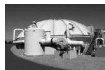
Provincetown Wastewater Treatment Plant Massachusetts, USA
