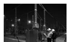
Brendale Substation Queensland, Australia
