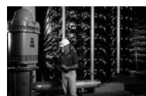
Water Treatment Membrane Plant Florida, USA
