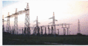
Rural Electrification Project, Ethiopia
